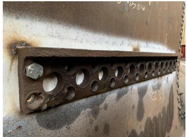
The support brackets are tack welded into place on the outer firebox.
