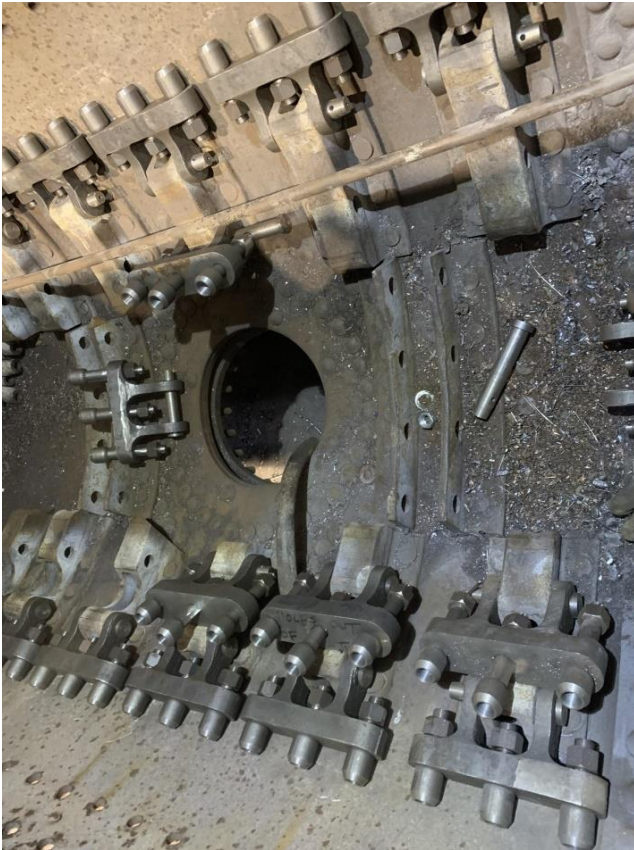
Looking up at inside of the top of the outer firebox where the crown sling hangers are being attached to the outer wrapper of the firebox, these will ultimately be attached to the crown stays on the top of the inner firebox and need to be in exactly the right location.
